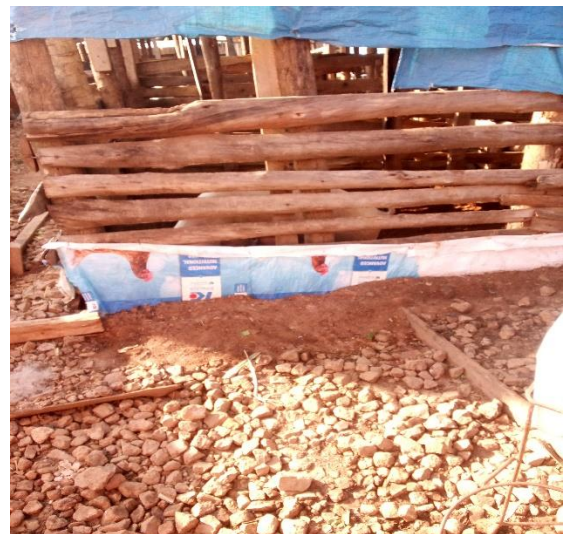
Figure 11. The apprentice mitigating floods on the piggery structure
