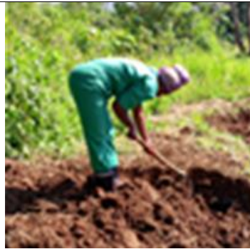
Figure 26 showing the intern digging the soil for brick laying to be used in the construction of Kyankorogoto parents P/S
